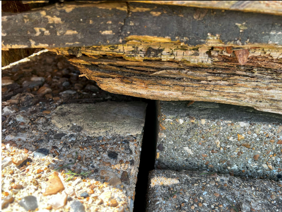
Rotten Timber Beam Bearing
