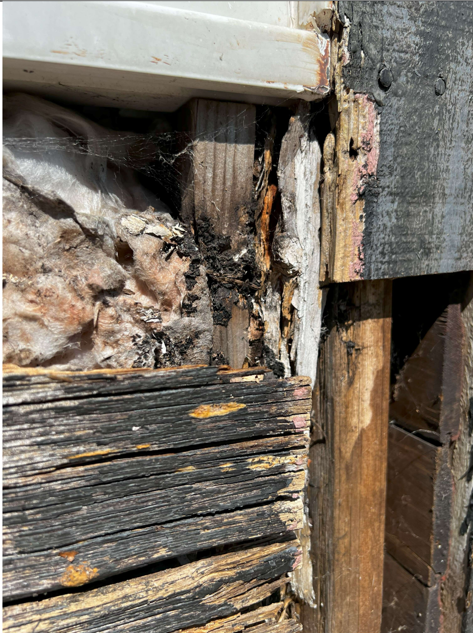
'Cladding 2' Rotten Timbers
