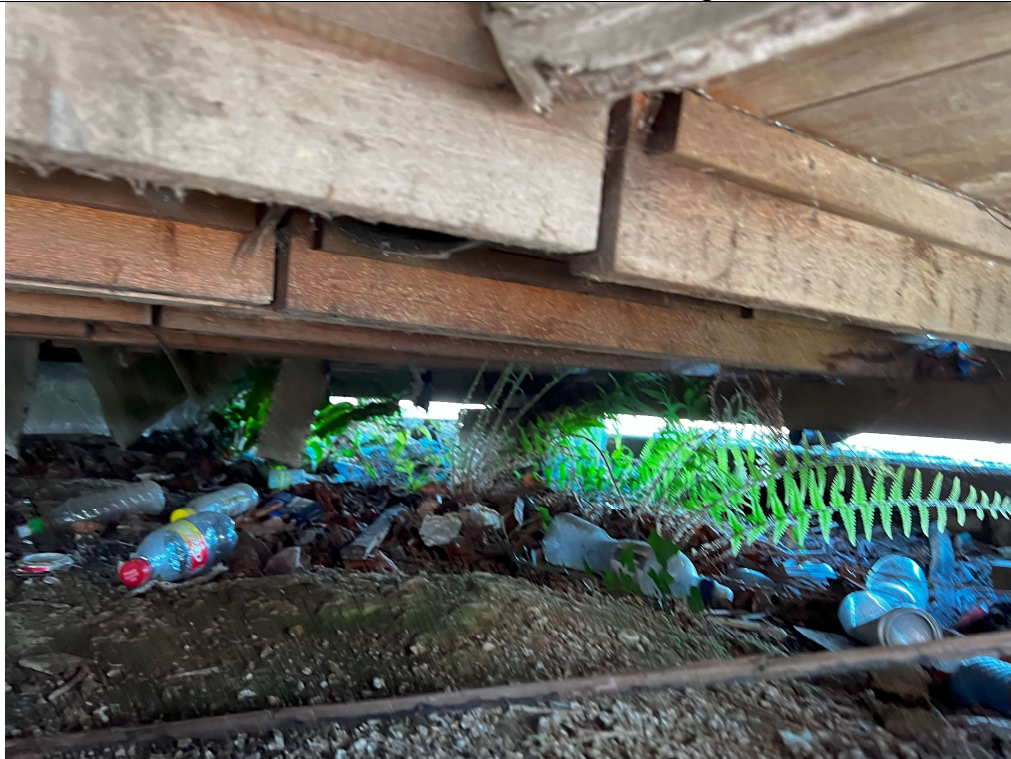
Incorrectly Installed Floor Joists
